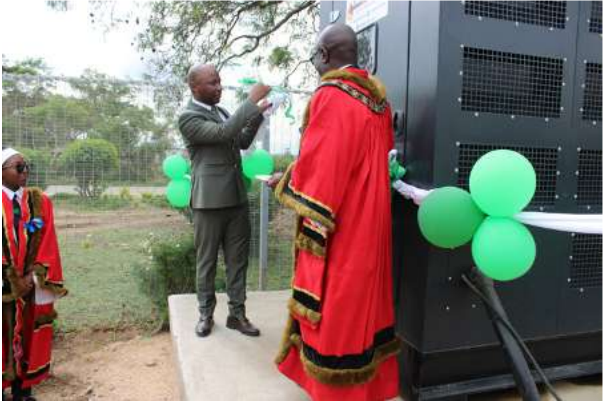
Minister of the State for Provincial Affairs and Devolution for Mashonaland East, Advocate Itayi Ndudzo, unveiling the new 550kva three-phase generator while the Mayor, Cllr C. Murova, looks on.
