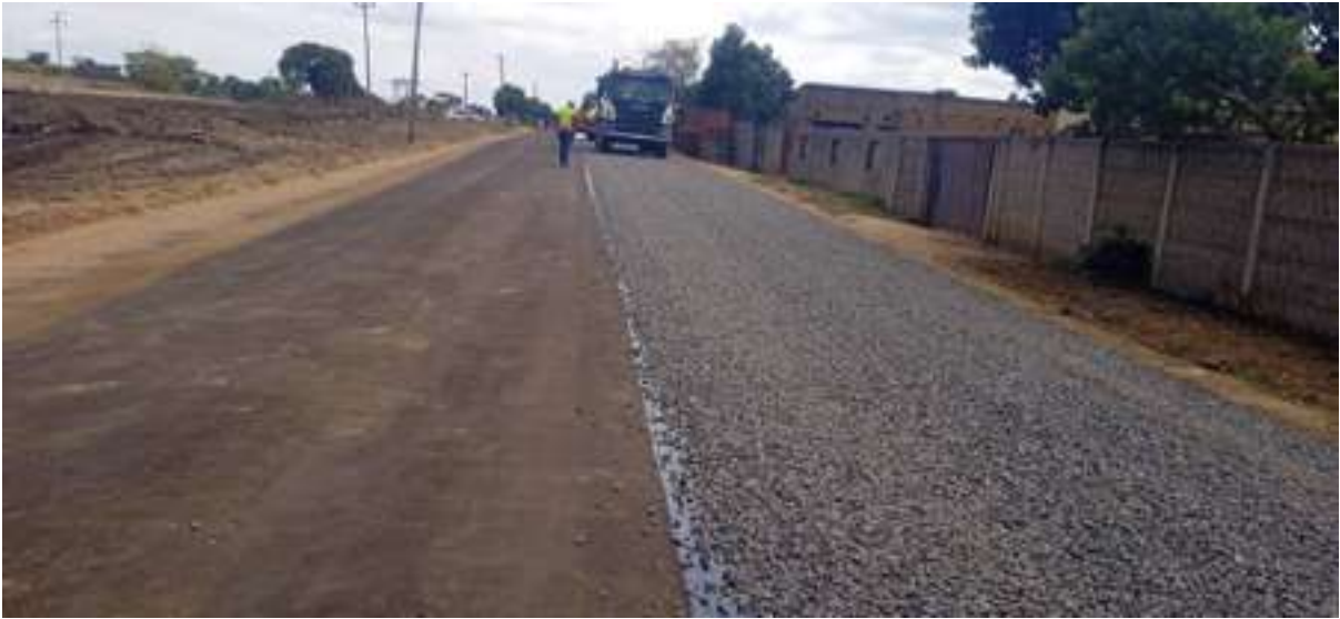
Morningside Crescent surfacing in the Morningside suburb
